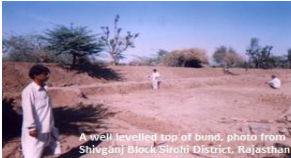
Plate 01: The level top of the structure maintained by the Flexi Tube Level
